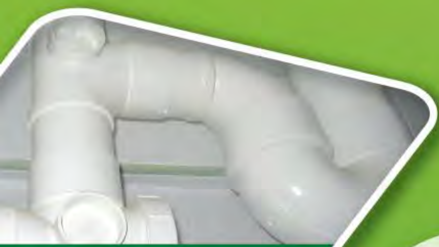
Waste Discharge Stack
