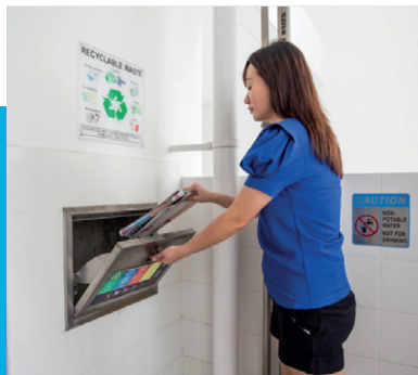
SEPARATE CHUTES FOR RECYCLABLE WASTE
