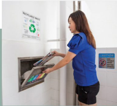
SEPARATE CHUTES FOR RECYCLABLE WASTE
