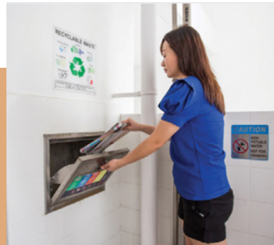
SEPARATE CHUTES FOR RECYCLABLE WASTE
