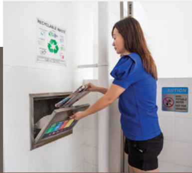
SEPARATE CHUTES FOR RECYCLABLE WASTE
