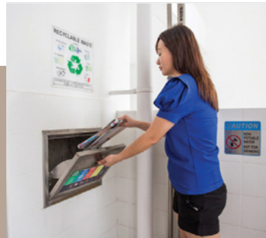
SEPARATE CHUTES FOR RECYCLABLE WASTE
