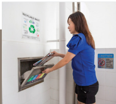
SEPARATE CHUTES FOR RECYCLABLE WASTE
