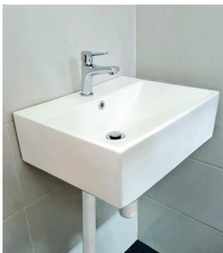
Wash basin with tap mixer
