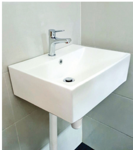
Wash basin with tap mixer
