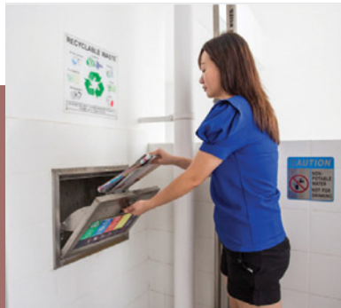
SEPARATE CHUTES FOR RECYCLABLE WASTE
