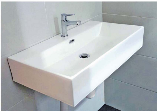
Wash basin with tap mixer in attached bathroom
