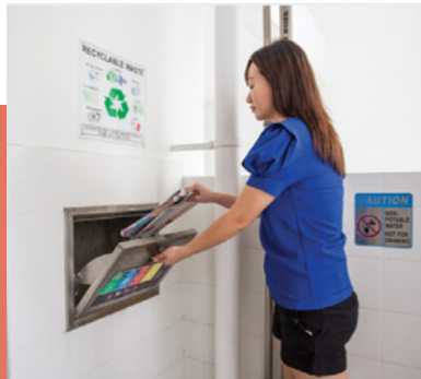
SEPARATE CHUTES FOR RECYCLABLE WASTE
