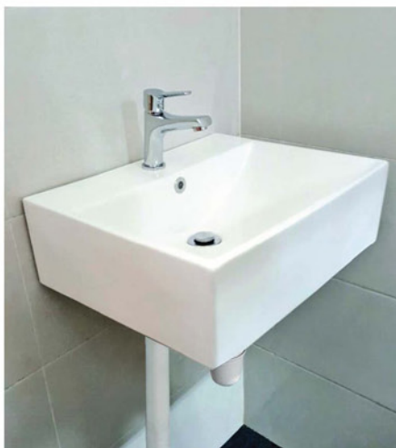
Wash basin with tap mixer
