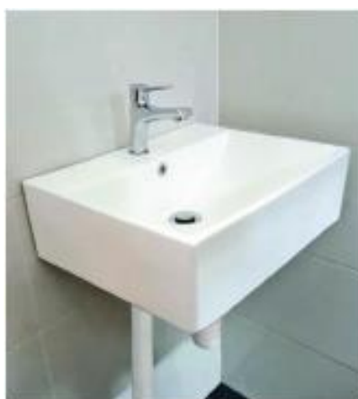
Wash basin with tap mixer
