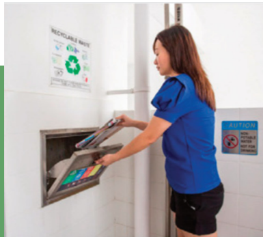
SEPARATE CHUTES FOR RECYCLABLE WASTE
