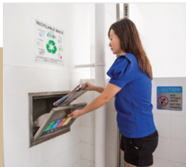
SEPARATE CHUTES FOR RECYCLABLE WASTE
