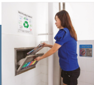
SEPARATE CHUTES FOR RECYCLABLE WASTE
